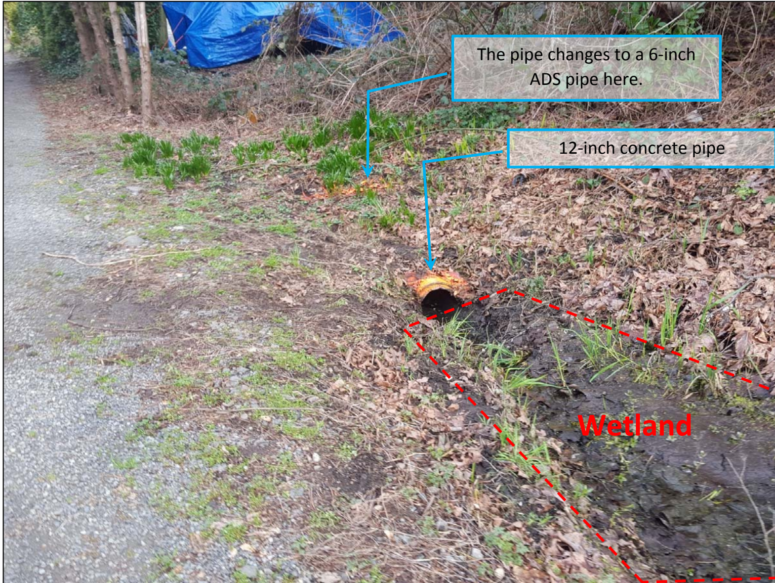
Picture 2 - The pipe changes from a 12-inch concrete pipe to a 6-inch ADS pipe. (Looking downward and northeast)
