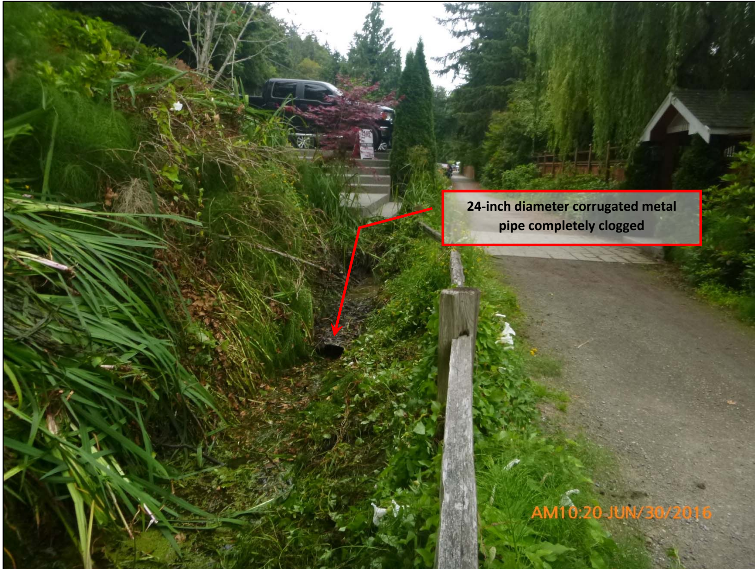
Picture 1 – This photo shows the clogged 24-inch corrugated metal pipe in front of the Hill residence. (Looking south)
