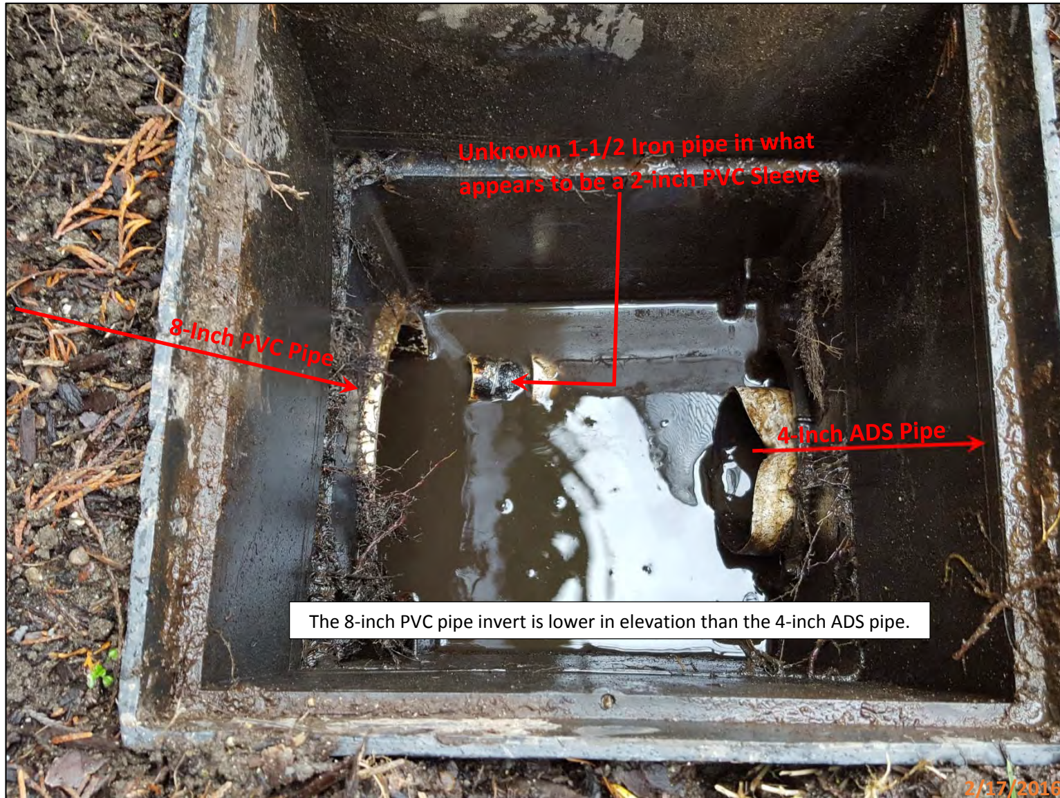
Picture 10 - This picture shows the yard drain after to the vacator truck cleaned it out. The 8-inch PVC pipe shown comes from the ELST trail drainage ditch. The 4-inch ADS pipe appears to be connects to a nearby homeowner drainage system to the east on East Lake Sammamish Shore Ln SE. The 4-inch ADS pipe was not cleared out or viewed with a pipe camera. This yard drain was completely filled with water to the rim of the structure prior to cleaning it out. See picture 9 to view this structure prior to it being cleaned out.
