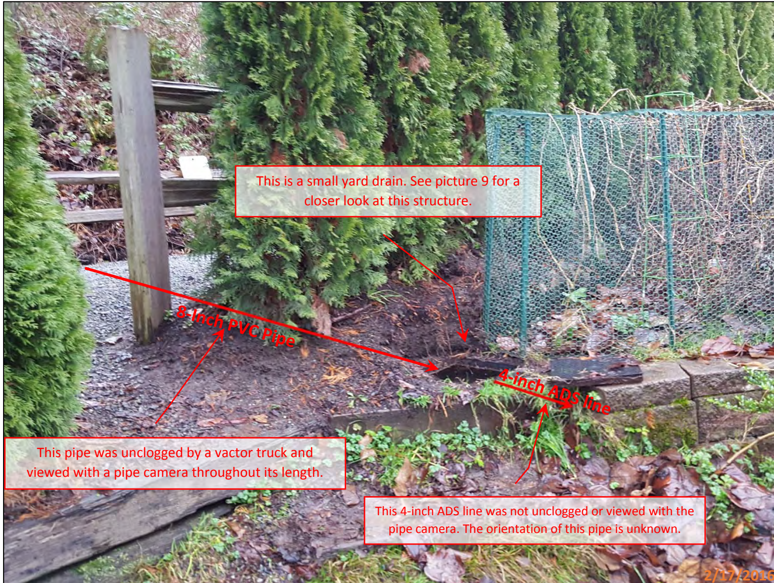
Picture 8 - This 8-inch PVC pipe travels west from the trail drainage ditch and enters a yard drain in front of 1428 E Lake Samm Shore Ln SE. This yard drain was filled to the rim with water prior to the vactor truck cleaning the structure out. This is the location that appears to overflow onto the adjacent private roadway in heavy rain events. This area received a complaint from the Tsilas Residence on 1/19/2016.
