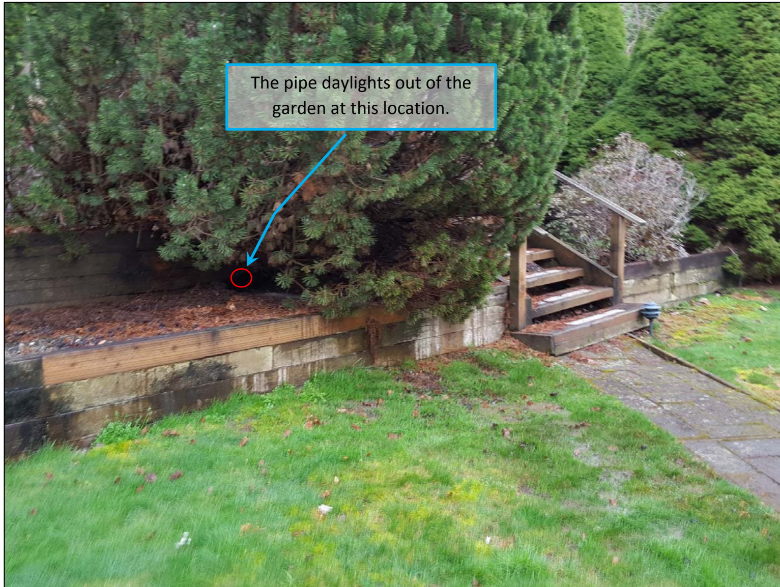
Picture 4 – Approximately 20' feet from the 90 degree bend on the east side of the trail, the pipe daylights out of the wood garden wall at 833 East Lake Sammamish Parkway NE. (Looking southeast)
