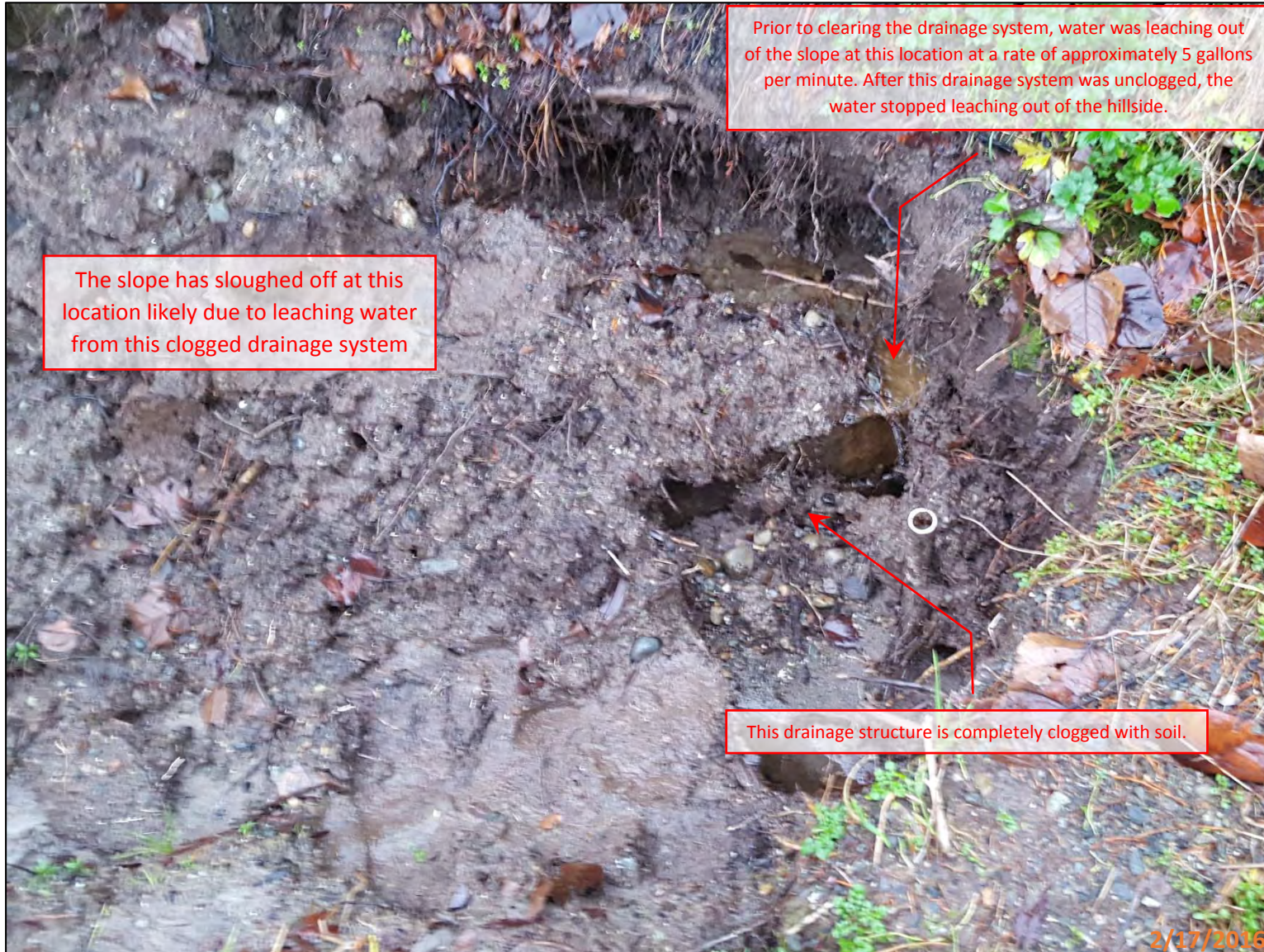
Picture 3 – This picture shows the clogged drainage structure in the trail drainage ditch adjacent to 1428 E lake Sammamish Shore Ln Se. (Looking downward and to the east)
