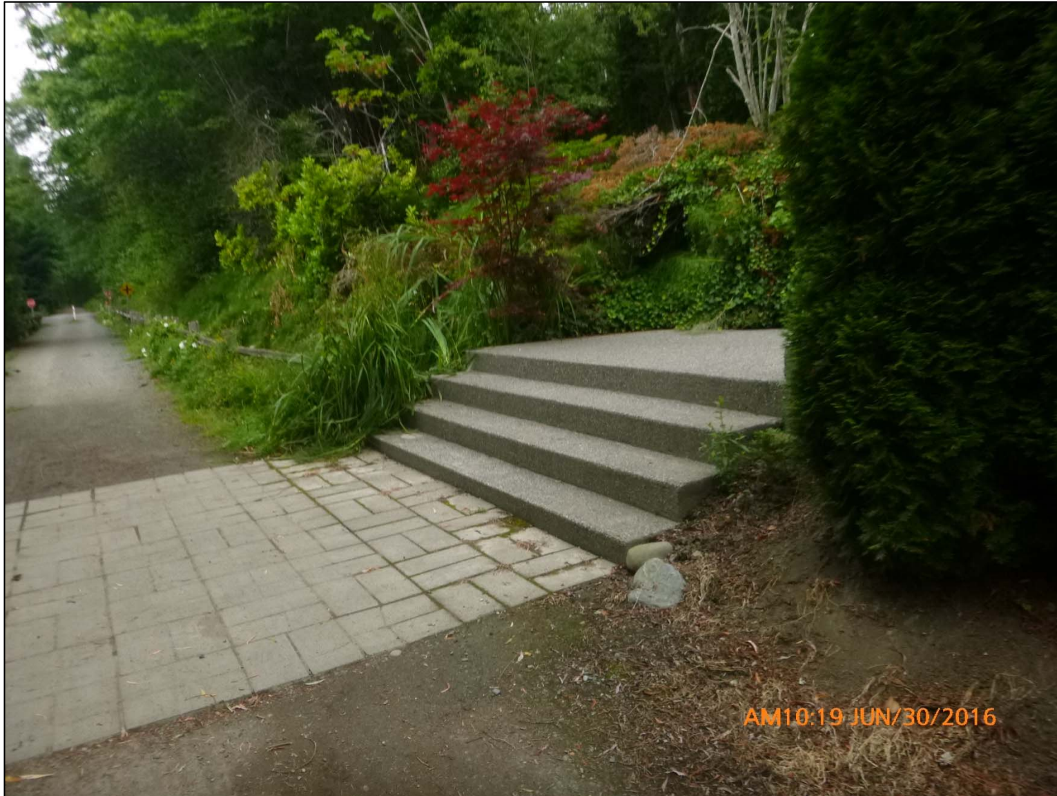
Picture 3 – Concrete stairs directly south of the clogged corrugated metal pipe. The pipe appears to travel southward under these stairs and towards the concrete rubble wall (Looking North)
