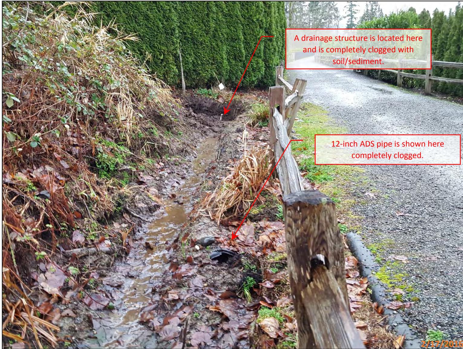
Picture 1 – This picture shows the drainage ditch on the east side of the East Lake Sammamish Trail. In this picture there is a clogged structure and a clogged 12-inch ADS pipe. This location was cleaned out with a vactor truck at a later time and subsequently viewed with a pipe camera. See picture 2 to see this location after the system was cleaned out. (Looking south on the trail adjacent to 1428 E Lake Samm Shore Ln SE)
