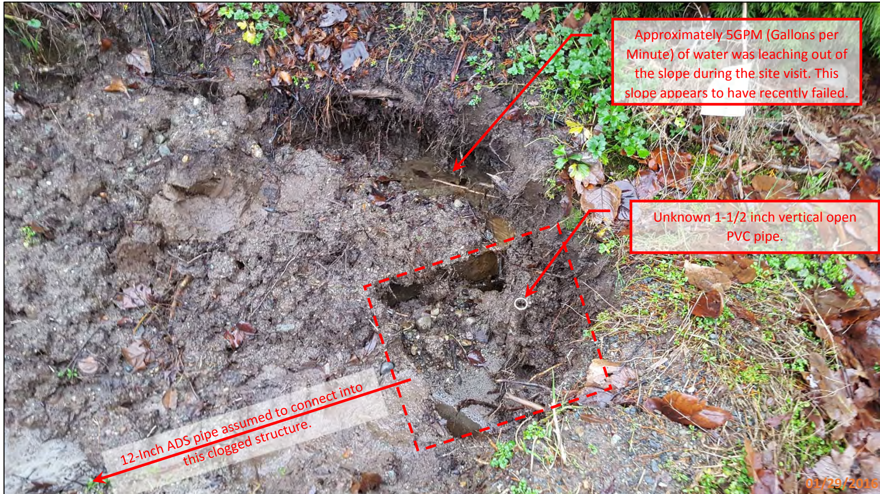
Picture 9 – This picture shows a clogged structure that connects to the 12-inch ADS pipe in the drainage ditch on the ELST trail. The slope adjacent and directly east of this structure has failed and clogged the ditch. There is also a minor amount of water leaching out/bubbling up out of the ground at this location. Note: There is also a 1-1/2 diameter PVC pipe sticking up vertically in the structure. This pipe is unknown.
