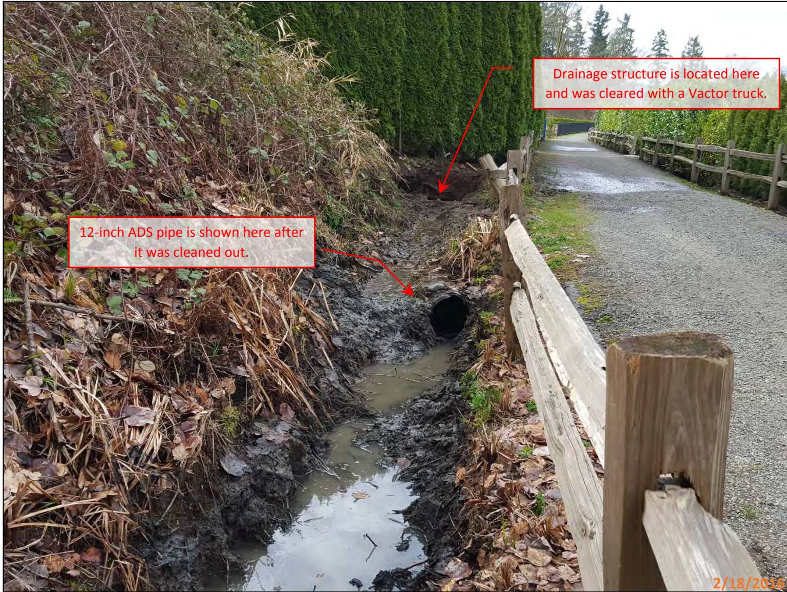
Picture 2 - This picture shows the drainage system from Picture 1 after it was cleared out with a vactor truck. This pipe is lower than the ditch which causes it to backflow. (Looking south on the trail adjacent to 1428 E Lake Samm Shore Ln SE)
