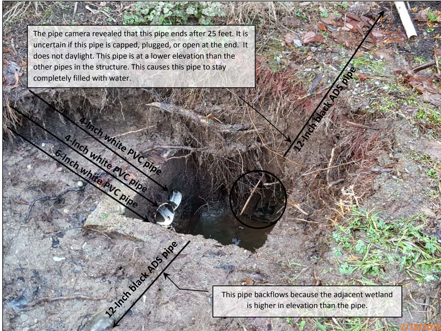
Picture 5 - This picture shows the drainage structure from Picture 3 after it was cleaned out with a vactor truck. The two 12-inch ADS pipes are not draining in the correct direction. The pipe on the right side of the picture ends after 25-feet resulting in the pipe being filled with water.
