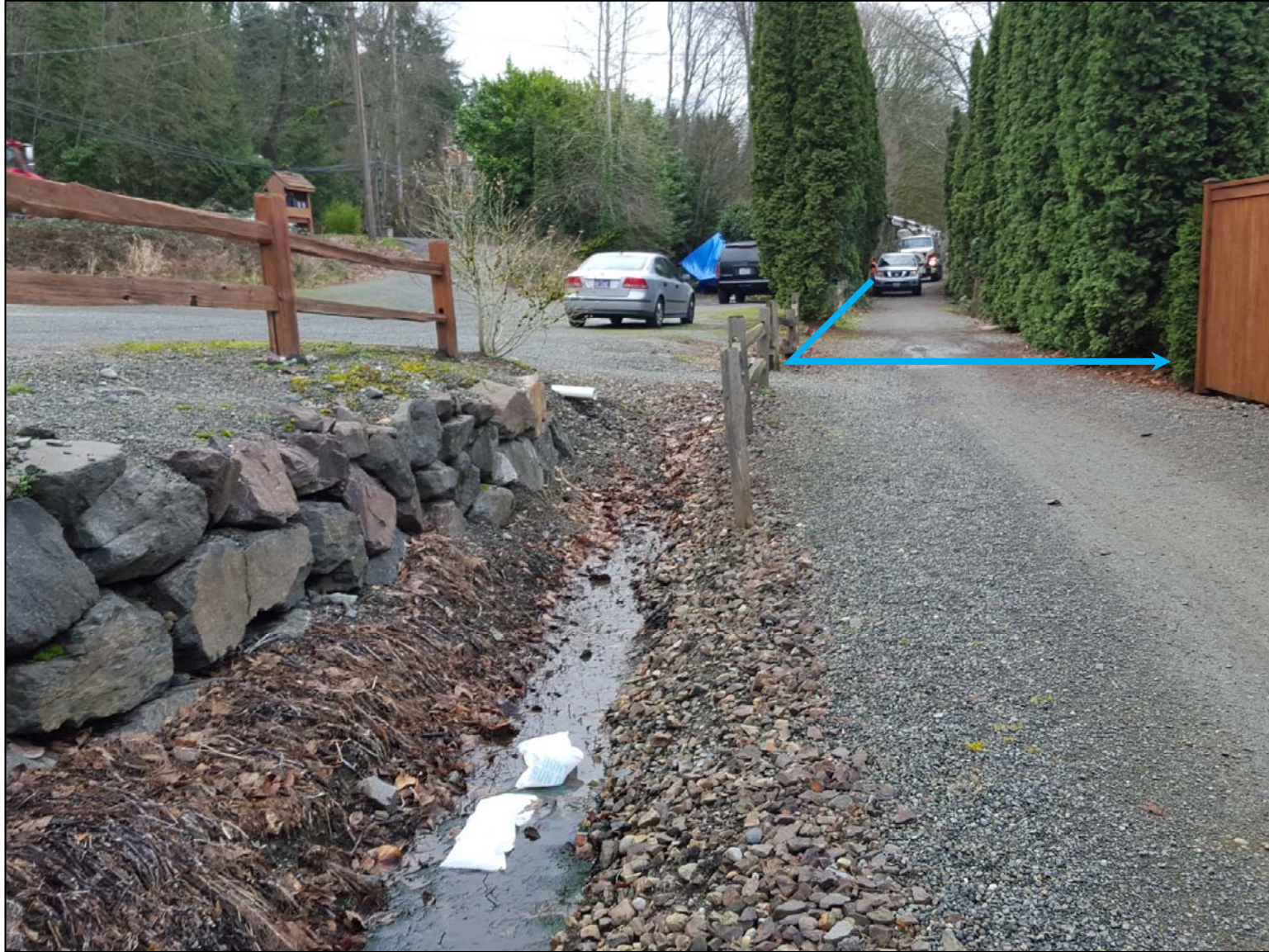
Picture 3 – Looking south towards the drainage line from Picture 1 and 2 (shown as blue line). The line takes a sudden 90 degree turn towards the lake. This picture was taken approximately 250 feet north of the beginning of the 12-inch concrete pipe from Picture 1. (Looking south)
