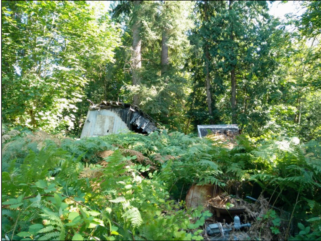
Figure 11. View of the partially burned and collapsed single-family residence; view is to the east.
