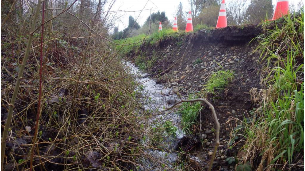
erosion is approximately 6 feet upstream from culvert entrance
