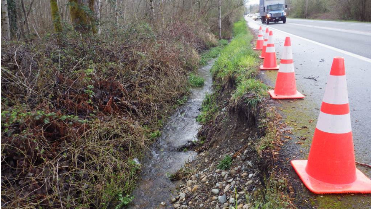
Erosion is occurring along approximately 30 feet of the stream channel.
