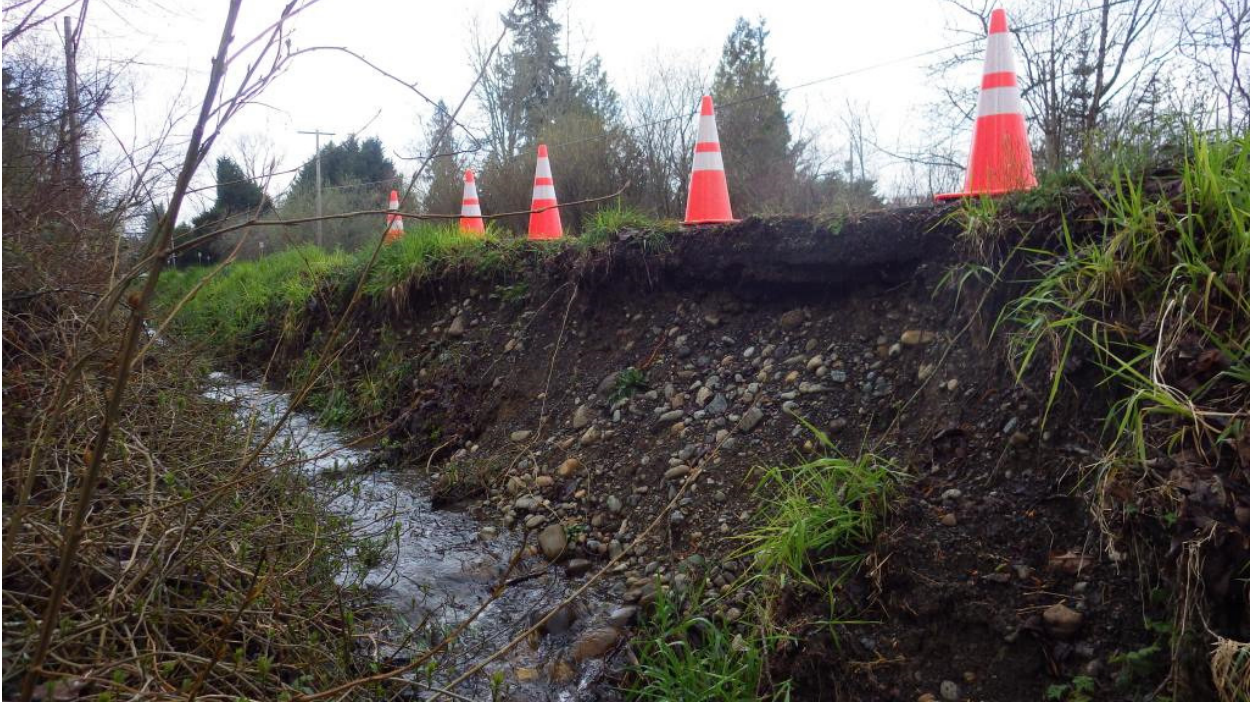
approximately 7 feet of asphalt is exposed; maximum undermine in center is 6 inches
