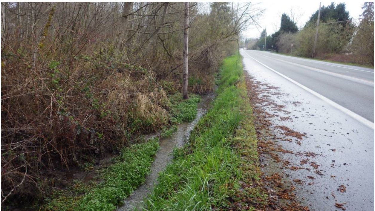
oversteepened bank extends upstream
