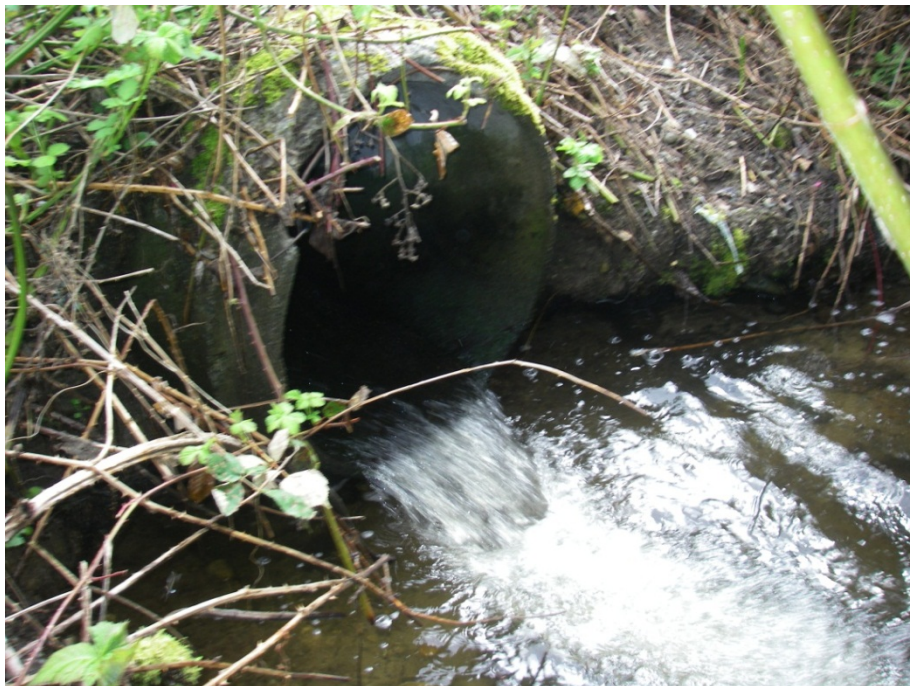
Figure 6. Drop at Downstream End of Culvert #3.
