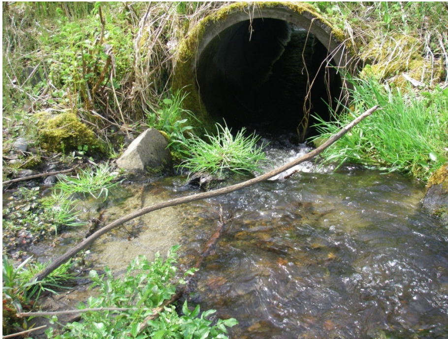
Figure 5. Steep Water Surface Drop into Entrance of Culvert #2 Caused by Bedload Buildup Upstream of Culvert Entrance.
