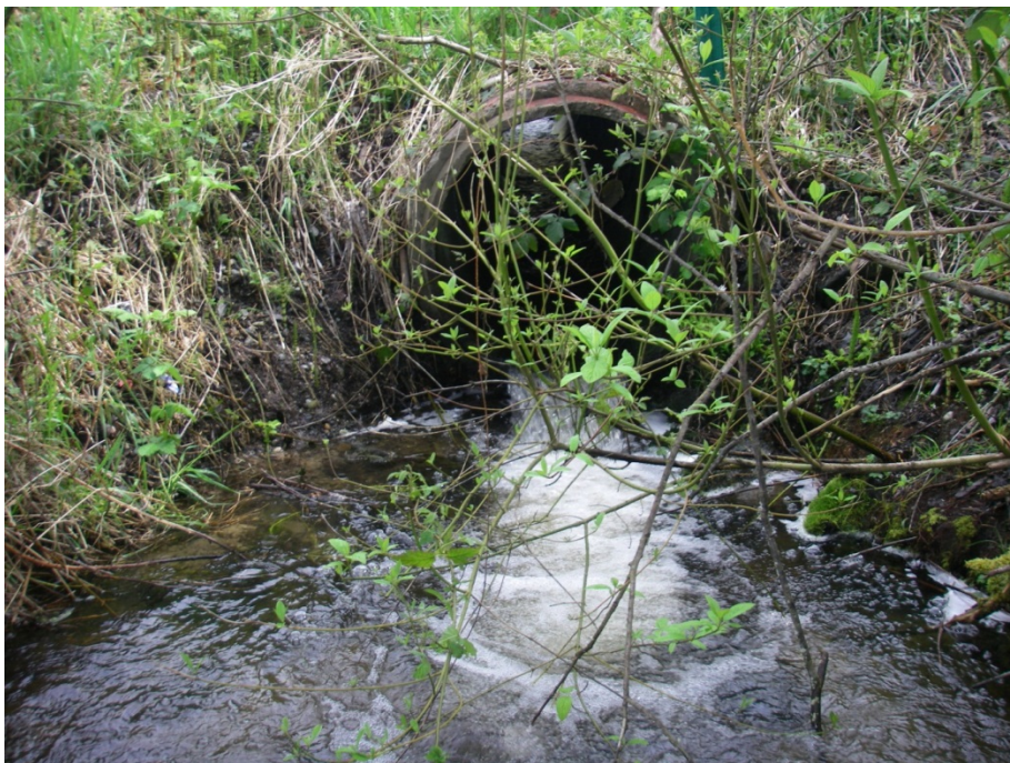
Figure 4. Drop at Downstream End of Culvert #2.
