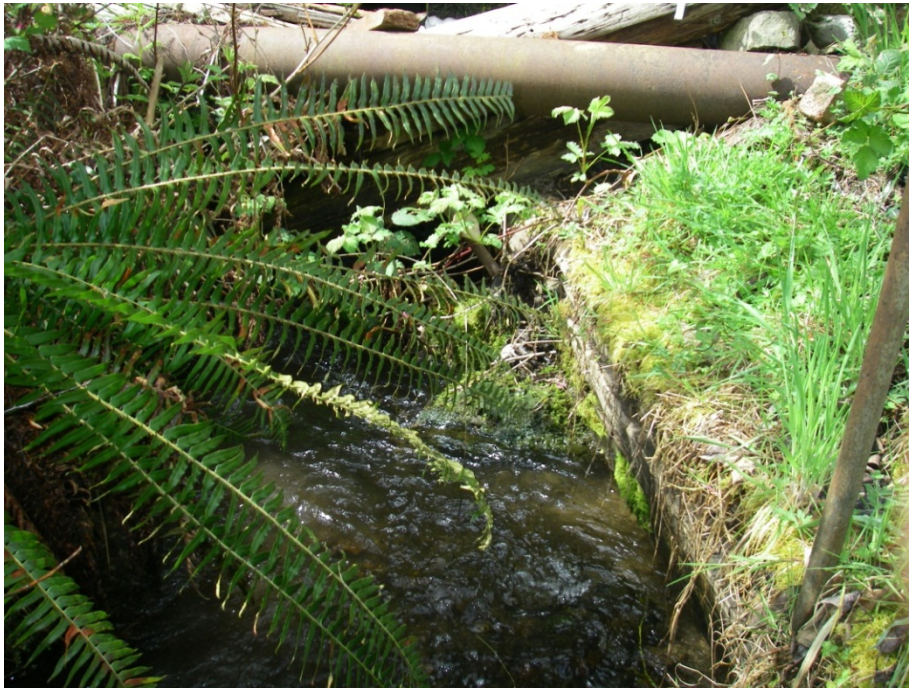
Figure 3. Broken Timber and Pipe Across Inlet to Culvert #1.
