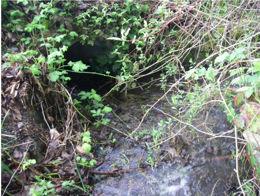
Figure 7. Zaccuse Creek Turns 90 Degrees from Drainage Ditch Along Parkway to Enter Culvert #3.
